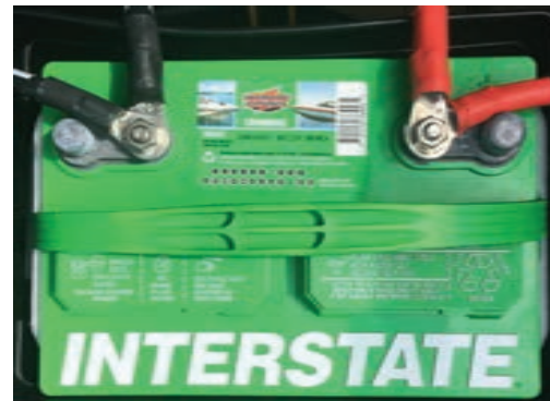
Battery post connections
